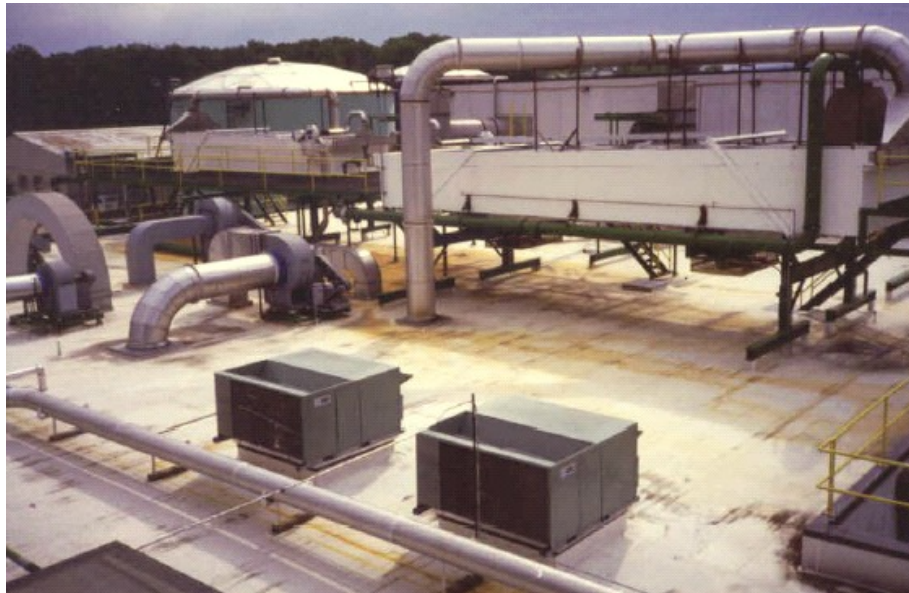
Figure 8. Air Condensers on Roof.
