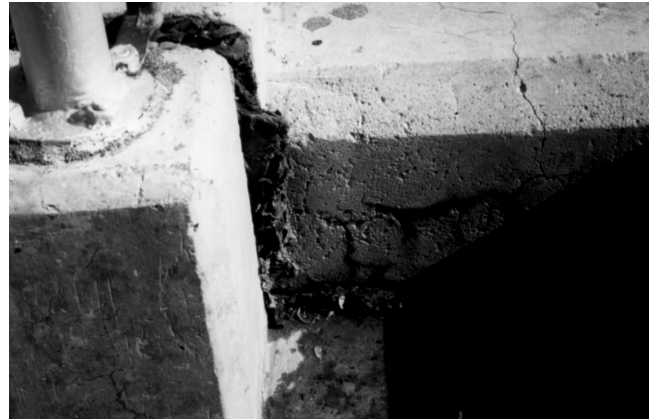
Fig. 5—Photograph showing closure of a joint and extrusion of joint-filling material due to ASR expansion.
