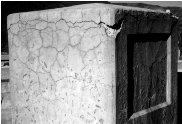
Fig. 2—Photograph of a parapet wall showing typical map-cracking at the surface.
