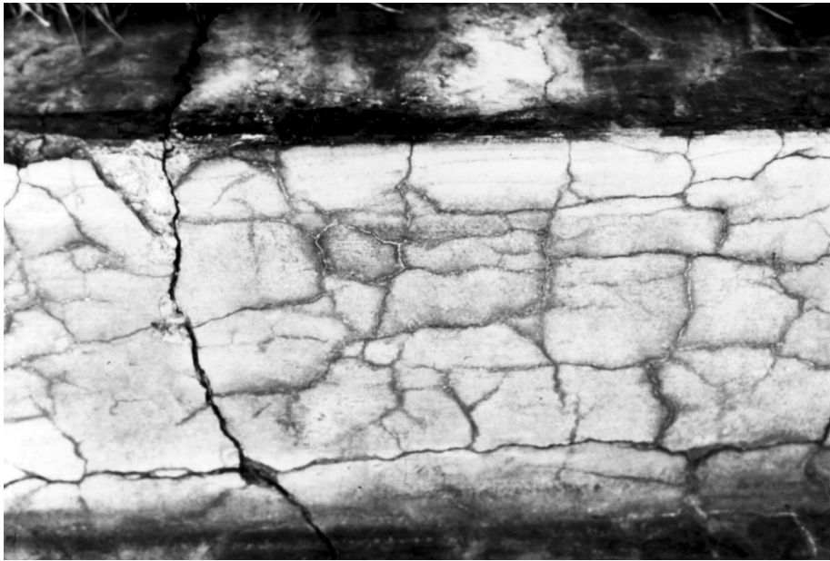
Fig. 8—Photograph of typical surface map-cracking due to ACR.
