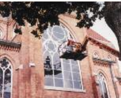
This window at Holy Rosary Chapel in Adrian, MI is being examined prior to the frame removal and reinstallation.
