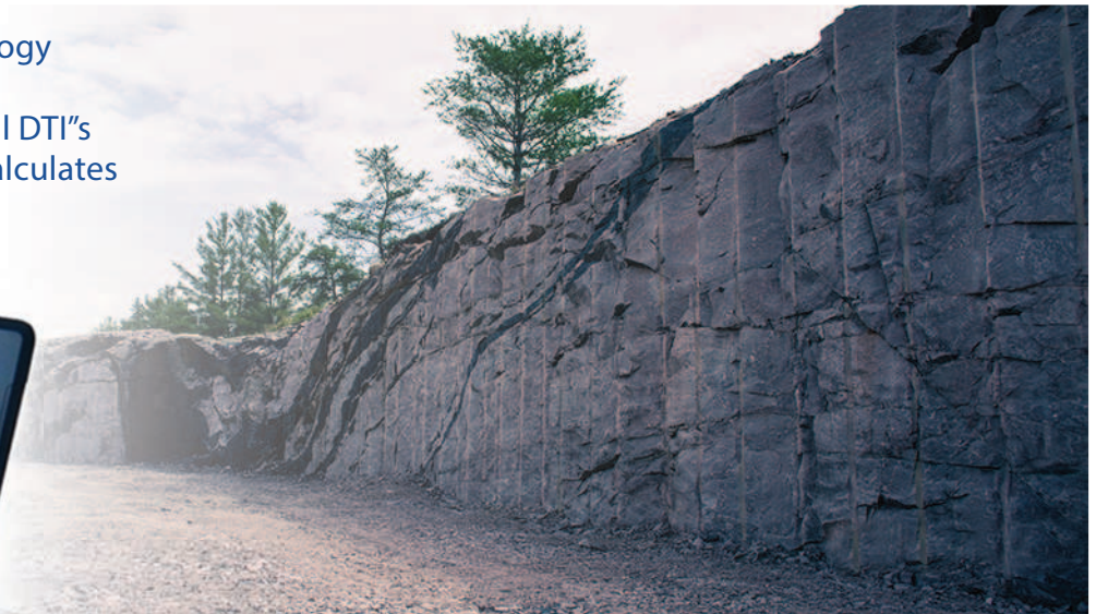
DTI’s AngleBlaster’s blasting results. All holes are parallel and in the same plain.
