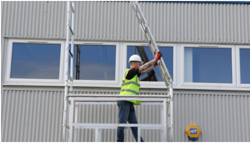
15. Continue erecting tower to final tower height repeating the AGR process as illustrated. Always ensure there is side protection to prevent falls. Platforms should be every 2m complete with handrails.
