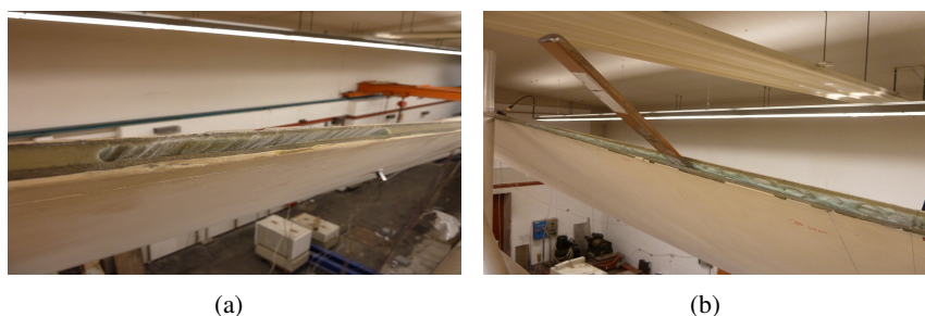
Figure 3 : Debonding introduced in the trailing edge of an SSP 34 m blade. (a) Original drilled debonding. (b) Extended debonding.
