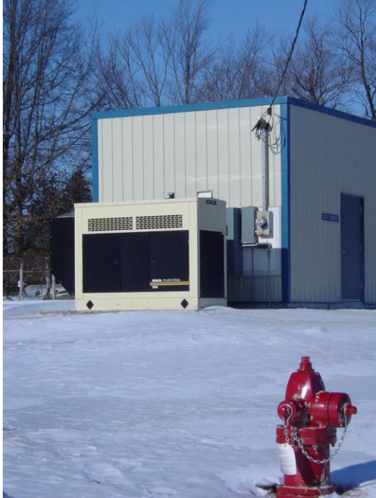
Emergency Generator outside Treatment Plant and New Hydrant
