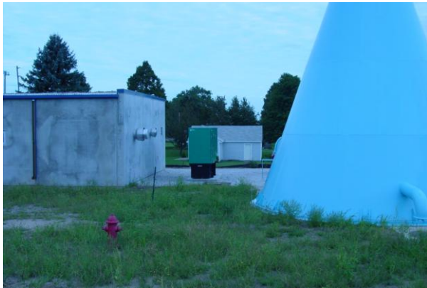
New hydrant, emergency generator, & elevated storage tower
