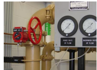
Filter control panel
