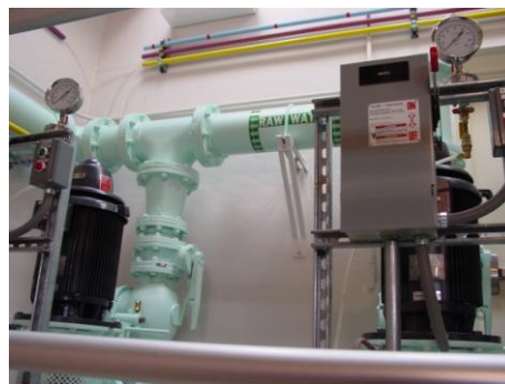
Vertical turbine well pump with flow meter
