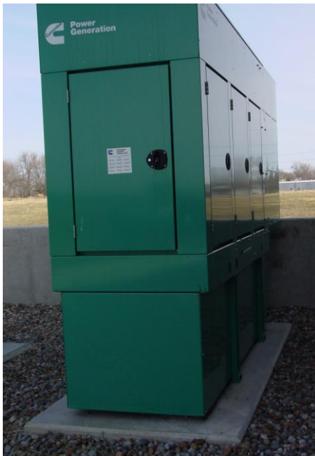
Emergency power generator
