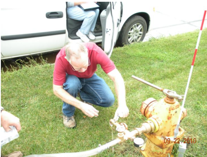
Multi-state AWOP Training Event: Using a hydrant sampler for mapping the chlorine levels in the distribution system
