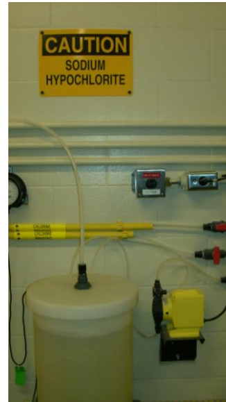
Liquid chlorine feed
