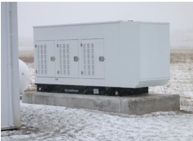
New emergency generator, to allow system to remain in operation during power outages.
