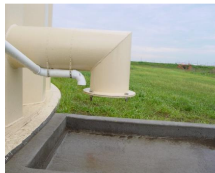
Major Monitoring & Reporting Violations
