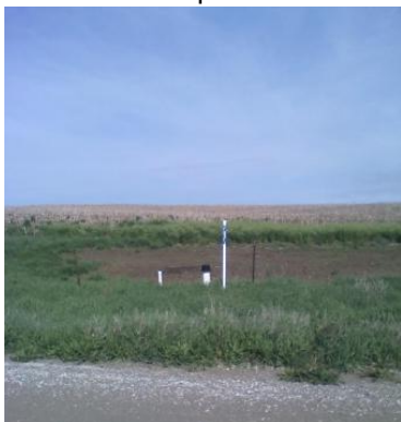
Example of a water main valve in a rural water system.
