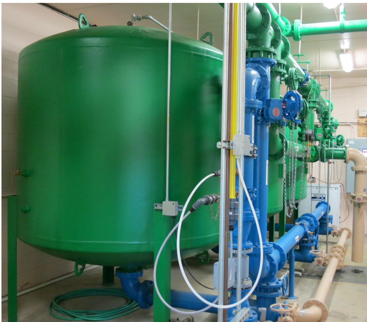
Pressure filters for removal of iron
