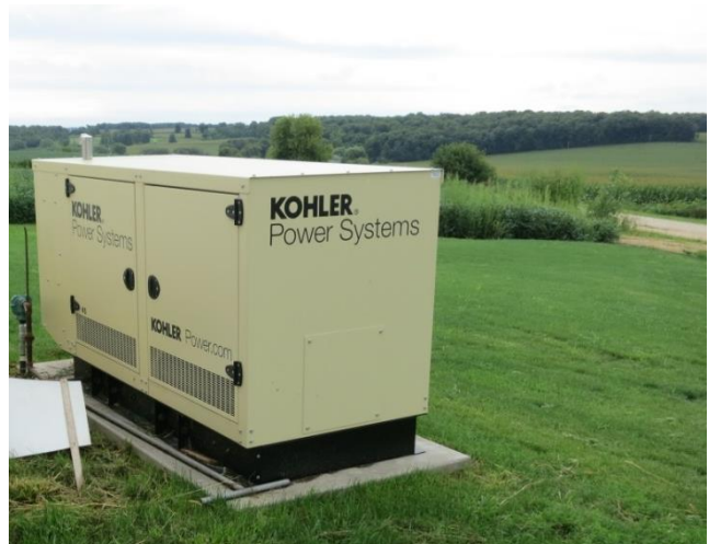
Emergency power generators
