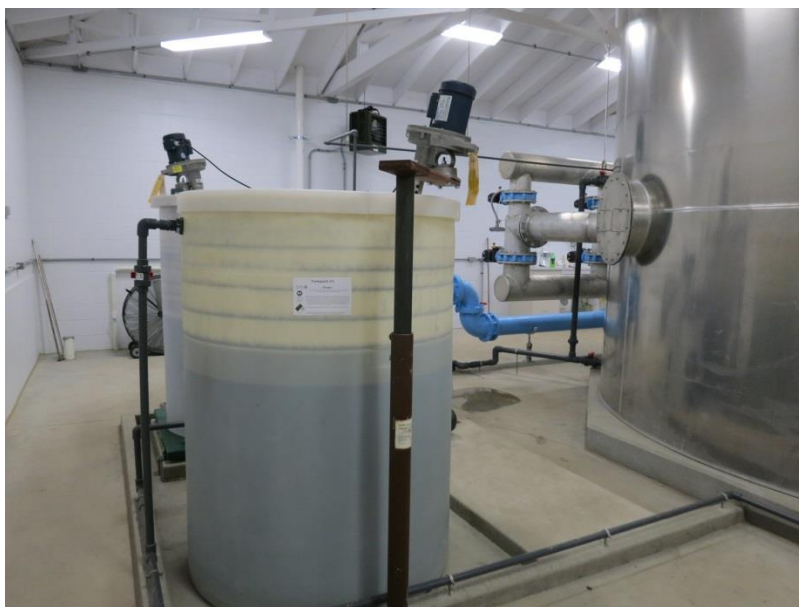
Hydrous manganese oxide feed for radium removal treatment
