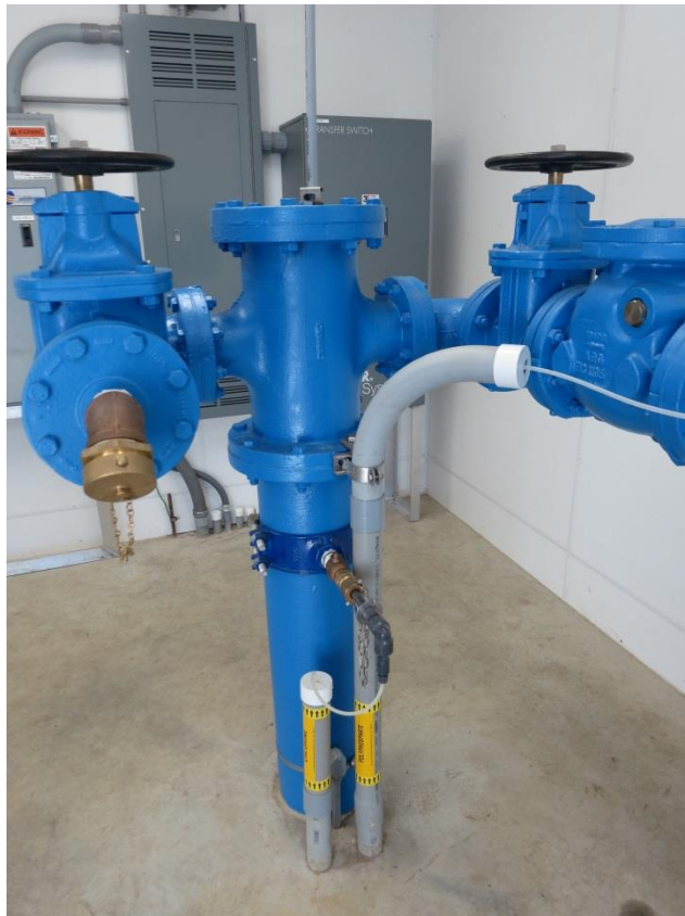
Chlorine and polyphosphate feedpoints on raw water line
