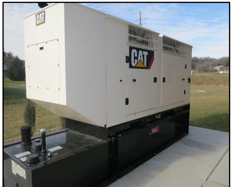
Emergency power generator
