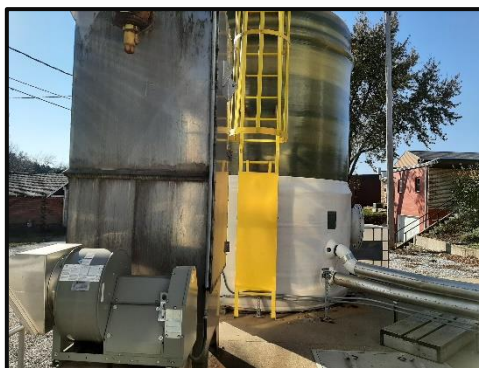
Major Monitoring & Reporting Violations
