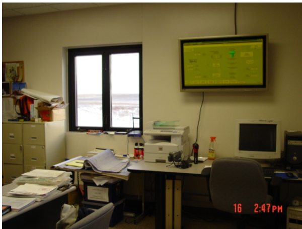
Office with computerized remote system-wide monitoring capability (typically called a SCADA system, or Supervisory Control And Data Acquisition system).
