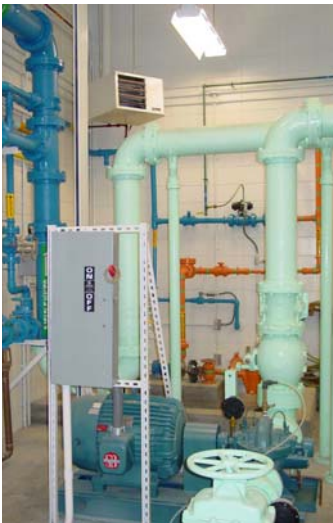
Pump & pipe gallery
