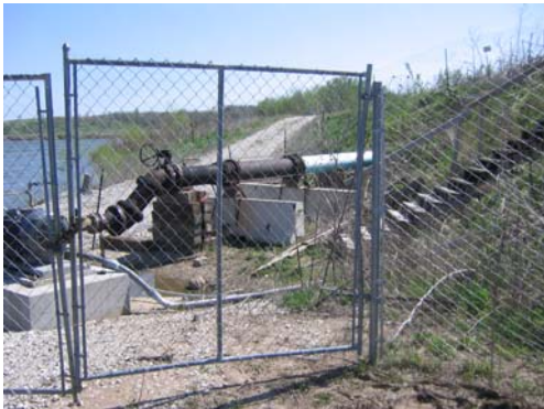
Raw water intake pump
