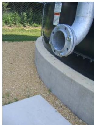
Storage reservoir overflow pipe and pad
