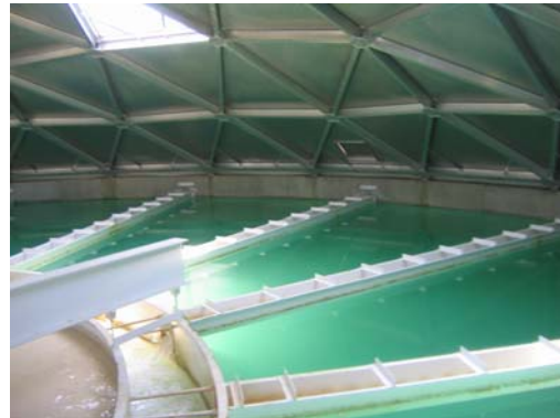
Lime softening basin and weir
