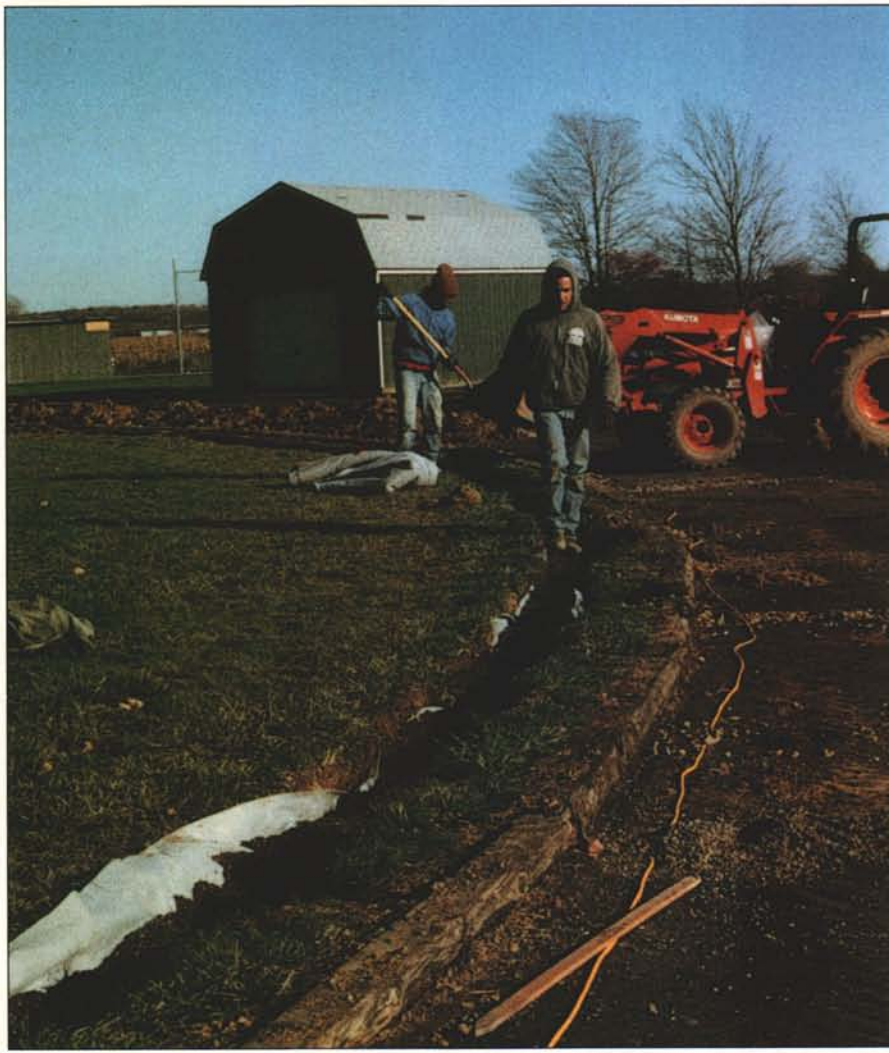
Installing a "sand drain" along the inside of a track can help to drain both the track and the field area inside.
