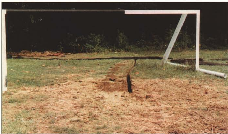
Strip drains can be used to target problem areas, like this one in front of a soccer goal.
