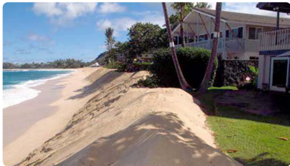
The image at top shows the restoration of dunes in progress on the North Shore of O’ahu; at bottom are the newly restored dunes that will protect homes from high waves. Source: Hawai’i Sea Grant.
