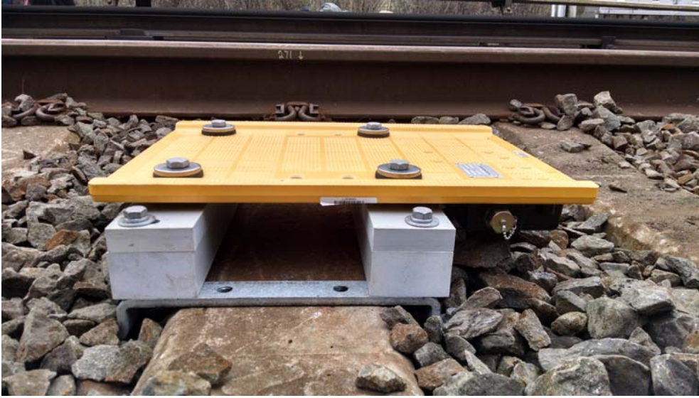
Transponder on Concrete Tie
