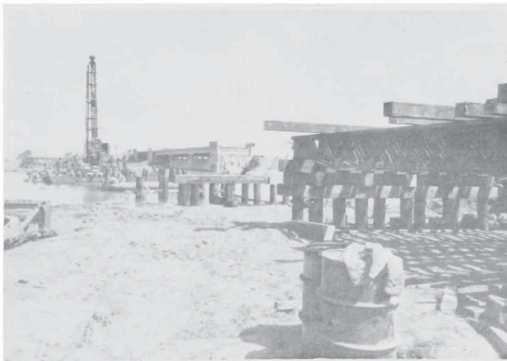
RAFT OF COMPANY "A", 85TH ENGINEERS, USED IN CONSTRUCTION OF 343RD ENGINEER BRIDGE NEAR ORBETELLO
