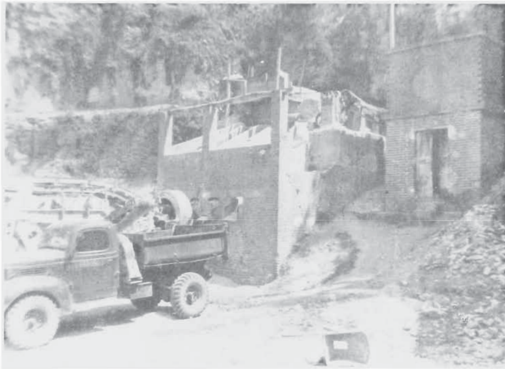
TRUCK OF BRITISH 3RD AIRFIELD CONSTRUCTION WAITING FOR A LOAD OF GRAVEL NEAR PIETRASANTA
