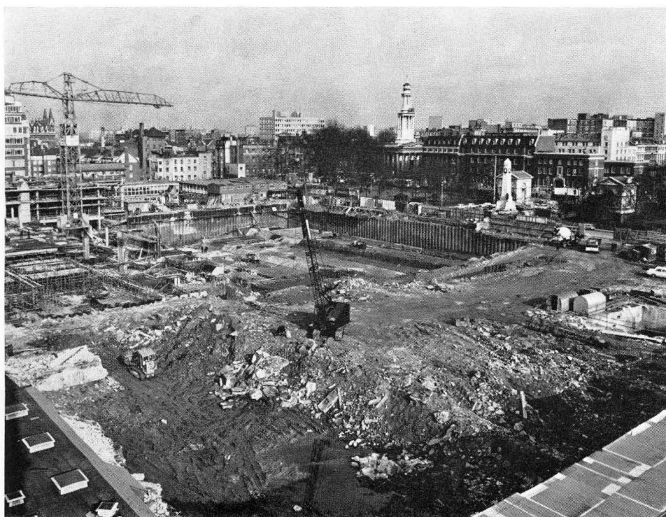
Both pictures show excavation work for reception and departure areas for cars and taxis
