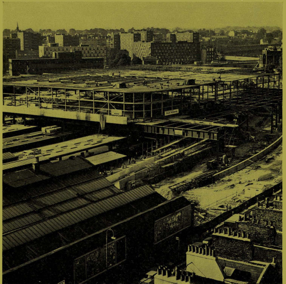
Partial construction of No. 1 platform and the parcels deck. The completed signal box and telecommunications centre can be seen in the background
