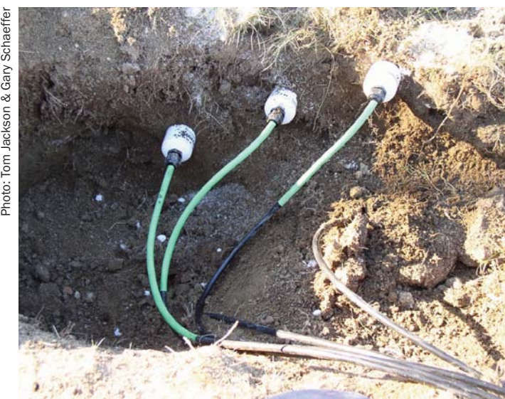
The pit in which the soil moisture probes have been installed to measure soil moisture over three different depths
