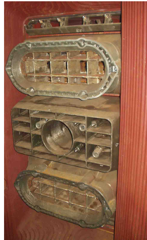
PM burner with vertical waterwall
