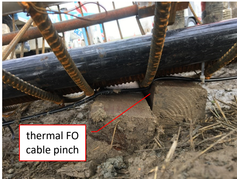
Figure 4-26: Thermal fiber optic cable pinched under reinforcement during handling prior to installation
