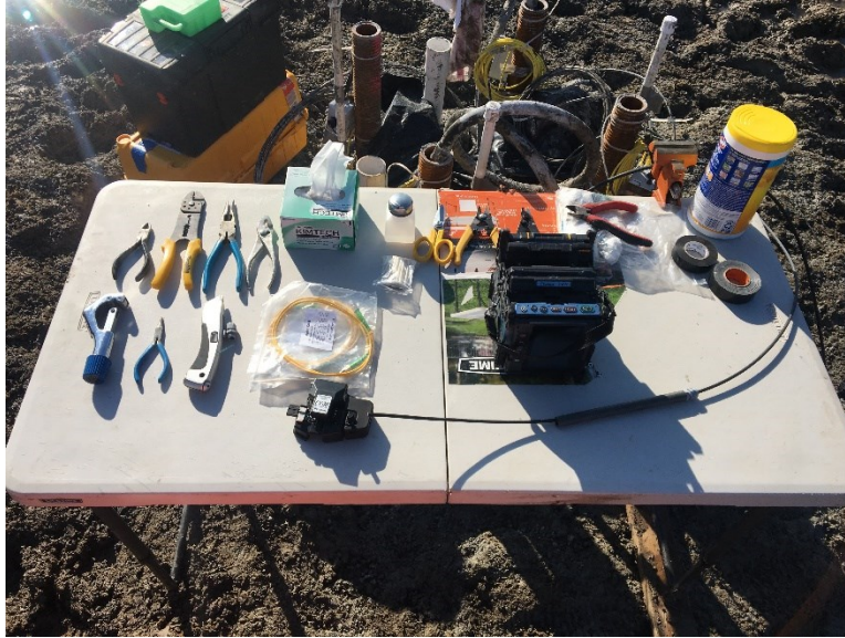
Figure 4-21: Photo of the field setup and tools used for splicing fiber optic cables from the piles
