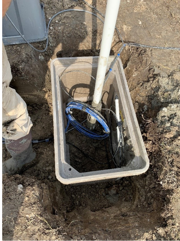
Figure 5-9: Enclosure vault used to protect the cable at the top of each borehole array
