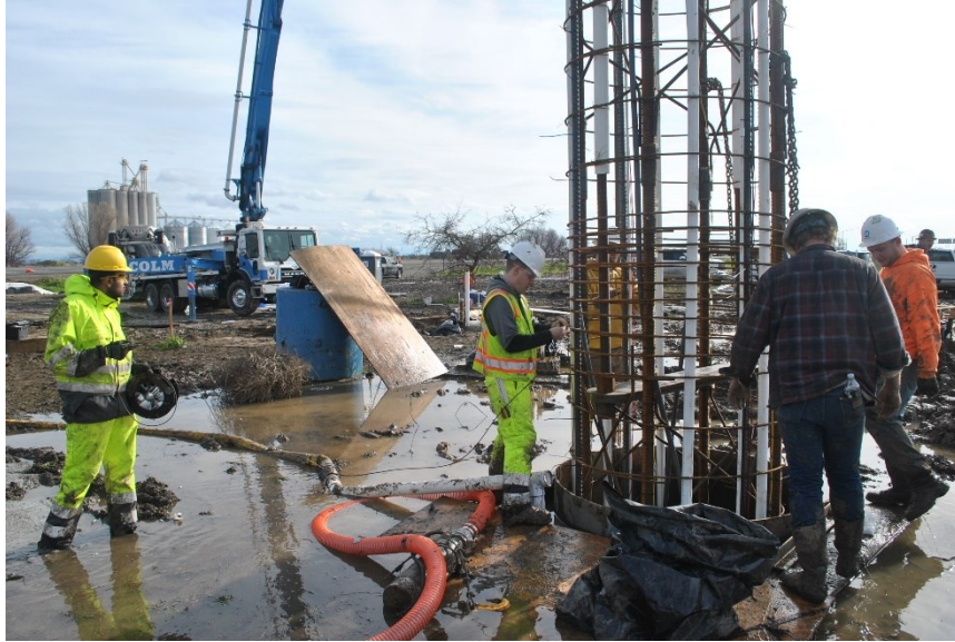
Figure 4-20: Installation of final fiber optic cable vertical during lowering of reinforcement cage
