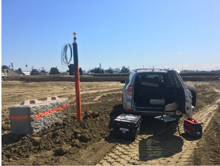
Figure 5-34: Standpipe riser, fiber optic cable, survey reflector, and fiber optic analyzer
