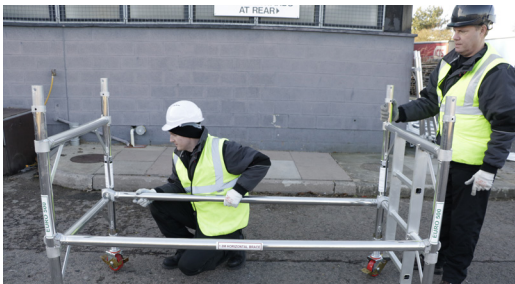
5. Fit another horizontal brace on the ladder side of the frames face down onto the 1st rung.
