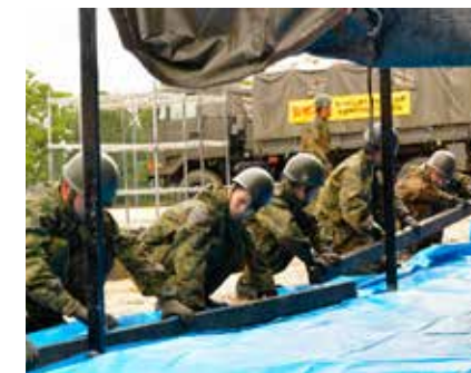
SDF personnel building a bathing facility following an earthquake whose epicenter was in Northern Osaka (June 2018)
