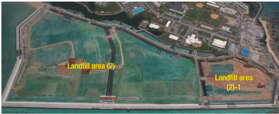
The progress of landfill construction in the waters south of Camp Schwab
