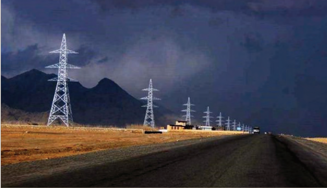
View of the electrical towers on the USAID-supported Arghandi to Ghazni Transmission Line. (USAID photo)
