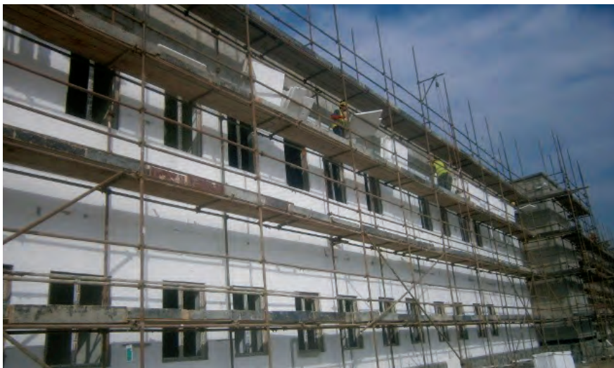
Construction of the Marshal Fahim National Defense University Joint Service Academy building in Kabul. (CSTC-A photo)
