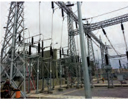
IRD provided quality-assurance services for this new power substation in Kandahar. IRD's contract with USAID was the subject of a SIGAR financial audit this quarter. (USAID photo)
