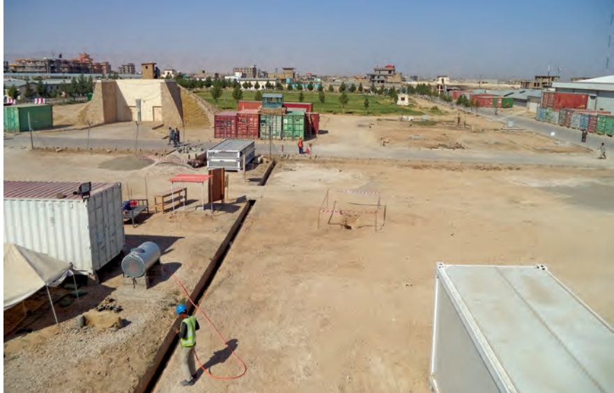
Construction continues on a women's compound at the ANP regional headquarters in Mazar-e Sharif, August 20, 2016. (USACE-TAA photo)
