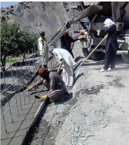
Workers install concrete for a highway project in southeast Afghanistan. (USAID photo)
