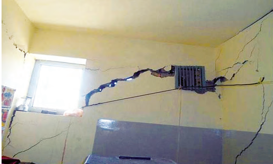
The crumbling interior of Building 17 , later demolished, at Baghlan Prison. (Bureau of International Narcotics and Law Enforcement Affairs photo)
