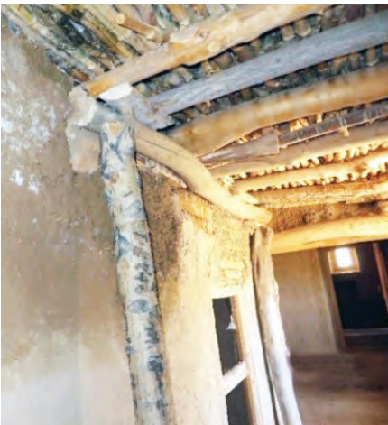
Leaking roof and saturated walls at a health facility in Ghazni Province. (SIGAR photo)
