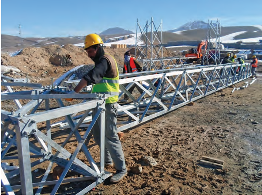
Workers assemble a tower for an electrical project to connect regional transmission systems. (USAID photo)
