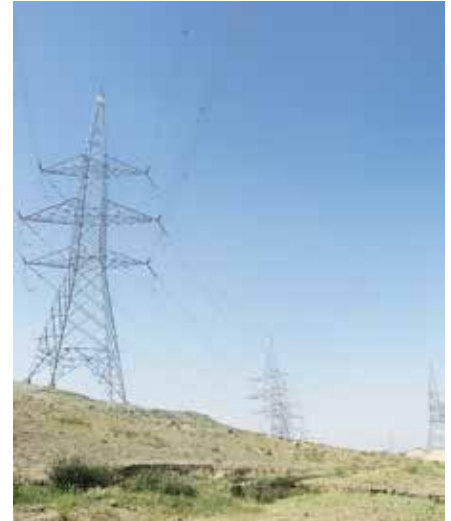
Transmission towers along the 76-mile-long Arghandi-Ghazni transmission line funded by USAID. (SIGAR photo)
