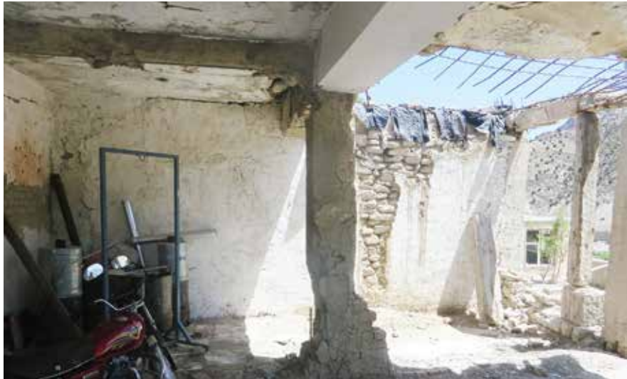
Structural damage at a clinic in Khost Province. (SIGAR photo)
