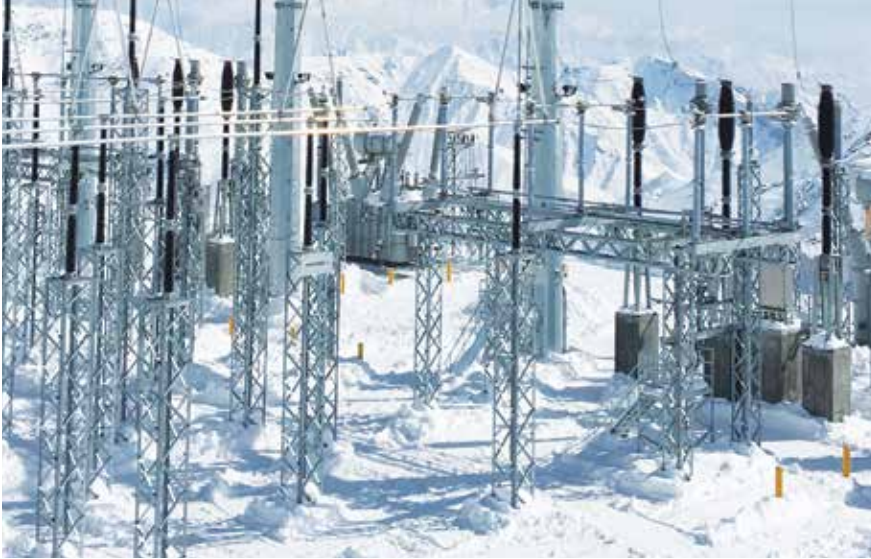
Power transformers and other infrastructure at the PTEC Salang substation. (SIGAR photo)
