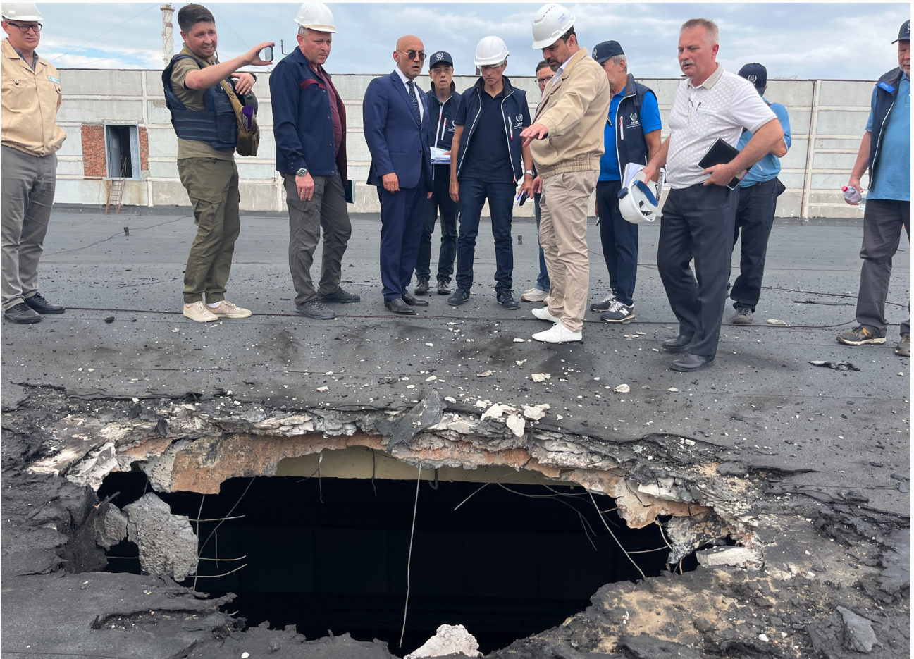
The IAEA team observes the damage caused by shelling on the roof of the special building at the ZNPP that houses, among other items, the fresh nuclear fuel and the solid radioactive waste storage facility. (Photo: IAEA)
