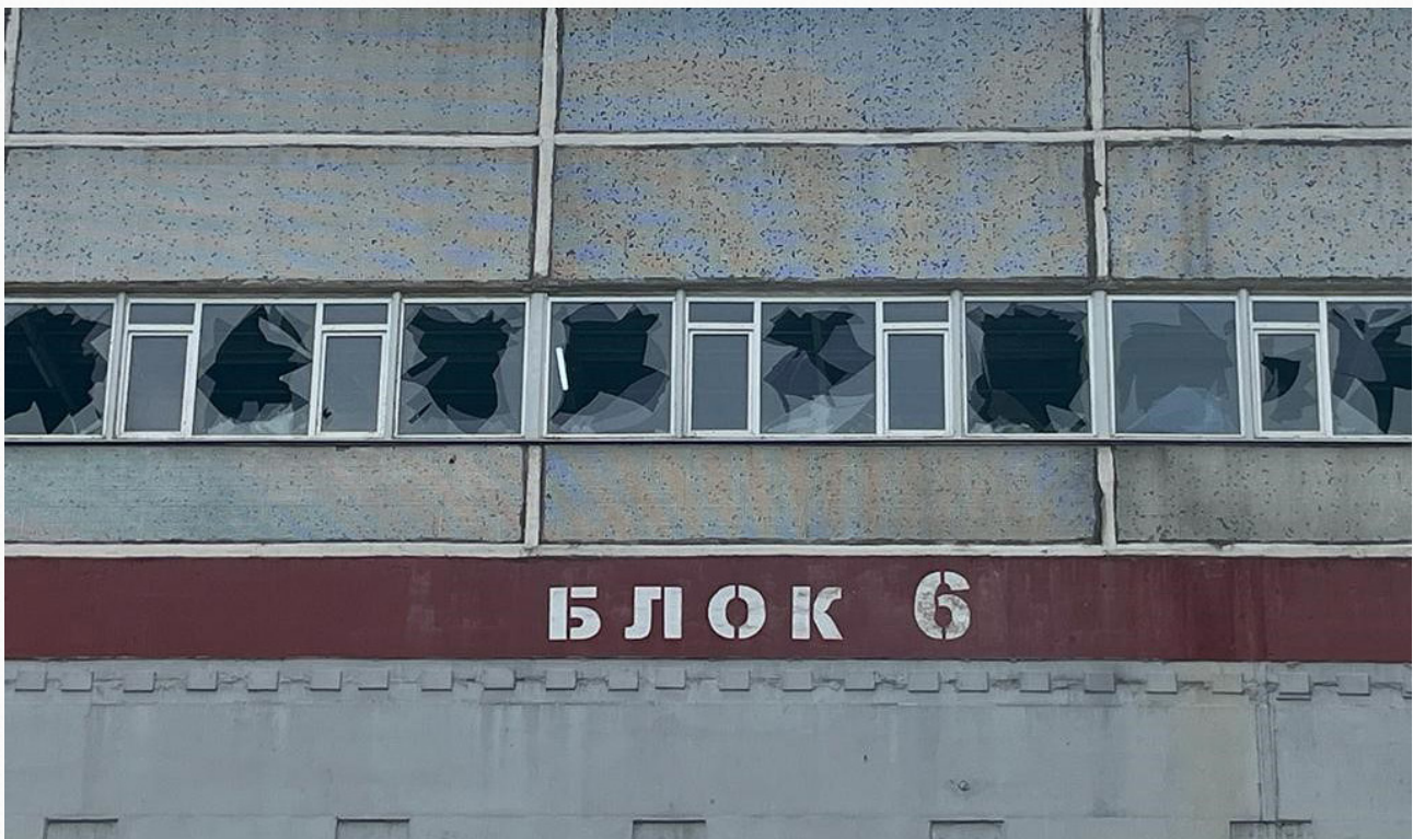
Damage caused by shelling to the elevated passage of Unit 6. (Photo: IAEA)
