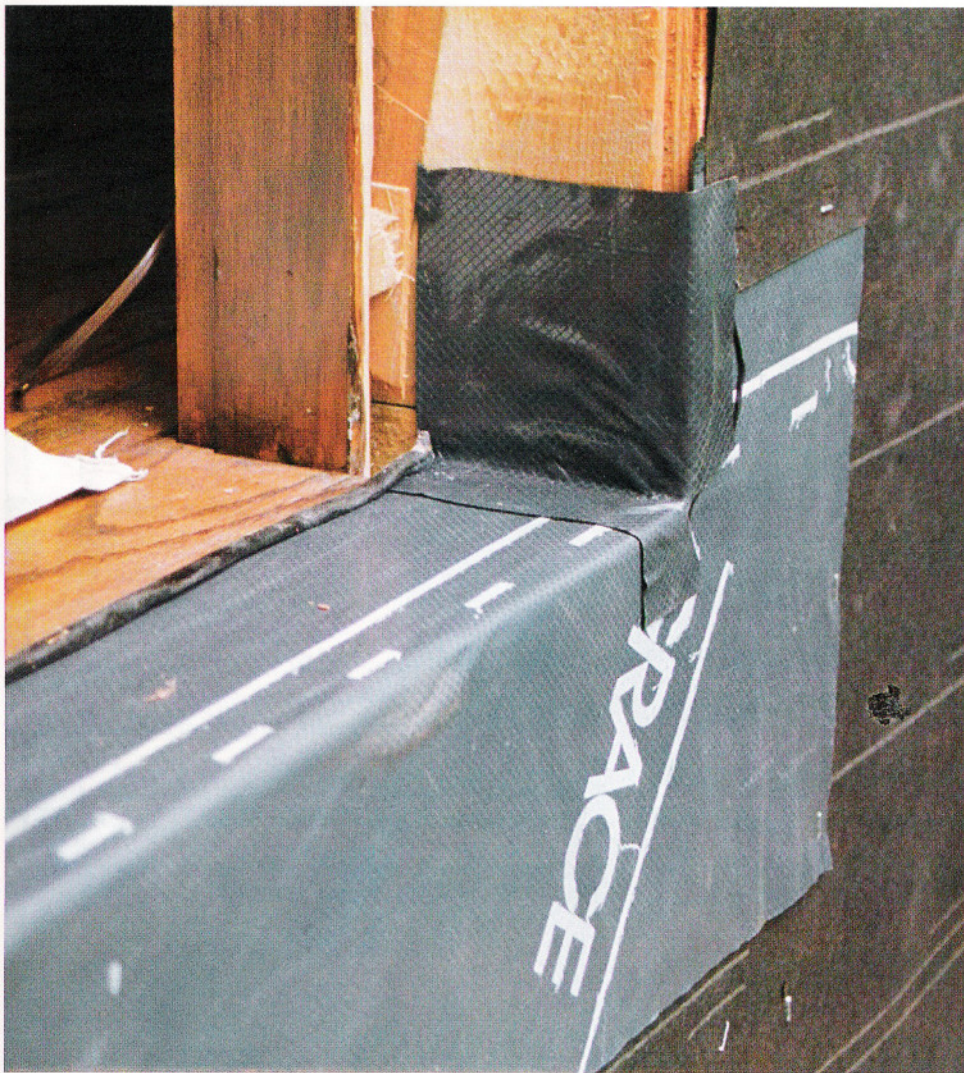
First, flash vulnerable spots such as rough sills to drain water. Note how the tar paper to the right of the opening laps over the top of the Ice & Water Shield flashing. In turn, the Ice & Water Shield laps the tar paper below.
