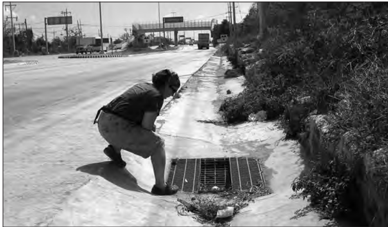
Patricia Beddows examines a highway drain that discharges directly into a cave in Puerto Aventuras. Aaron Addison.
