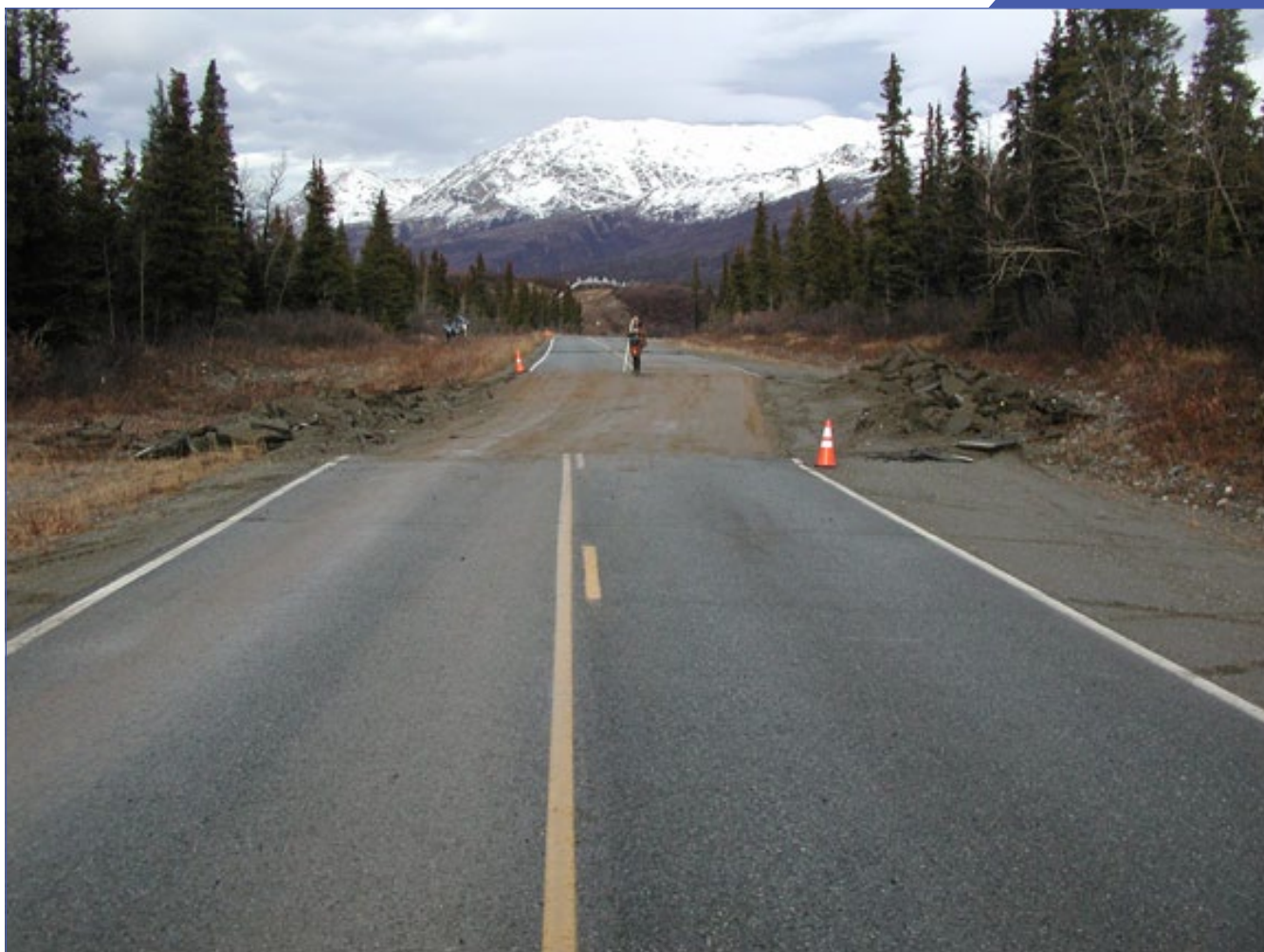
This segment of Alaska's Richardson Highway experienced an 8.5 foot lateral offset during the M7.9 Denali earthquake of November 3, 2002. This location is near where supports to the Trans Alaska Pipeline sustained damage. Image courtesy of the U.S. Geological Survey ( earthquake.usgs.gov/earthquakes/eqinthenews/2002/uslbb1 ).
