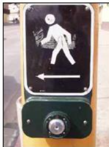
Figure 48: A pedestrian call button that gives audible and visible response when pressed
