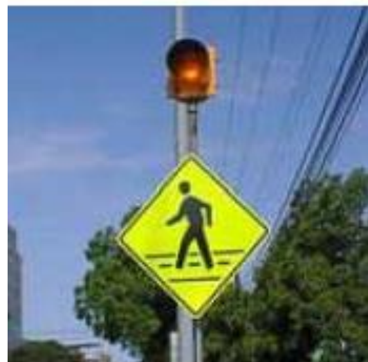
Figure 72: A flashing beacon used in conjunction with a pedestrian crossing sign in Austin, Texas
