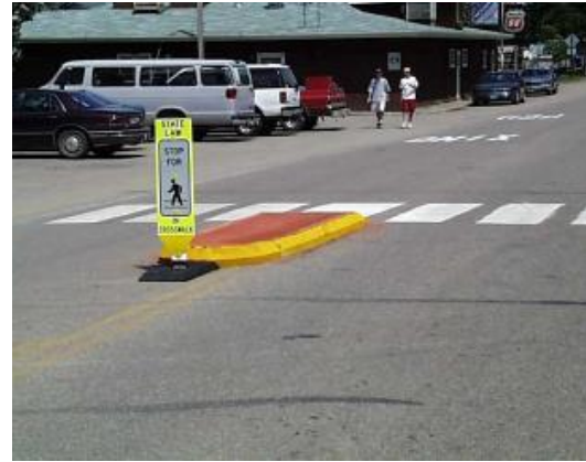
Figure 15: A removable pedestrian island installed in conjunction with an in-roadway yield to pedestrians sign at a crosswalk in Minnesota.
