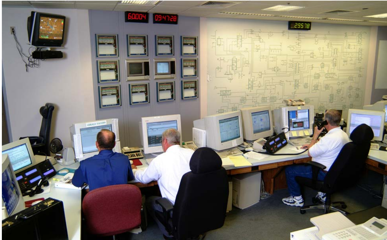
Figure 4.3. This photo highlights the key features of a control center. On the far right is a map. Although it is too small to show these details, the map indicates the location of power plants and transmission lines under the control of the center, usually with colored lights that indicate the status of the power plant or transmission line (e.g., red for out of service). Connections to adjacent control areas are also indicated. (Photo courtesy of Electric Reliability Council of Texas [ERCOT].)
