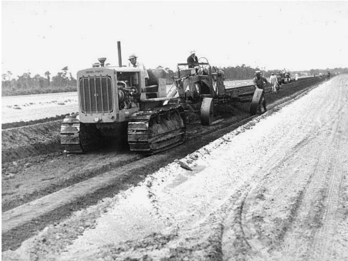
Figure 1. Construction Underway at the Malcolm McKinnon Airport, St. Simons Island, Glynn County, Georgia.
