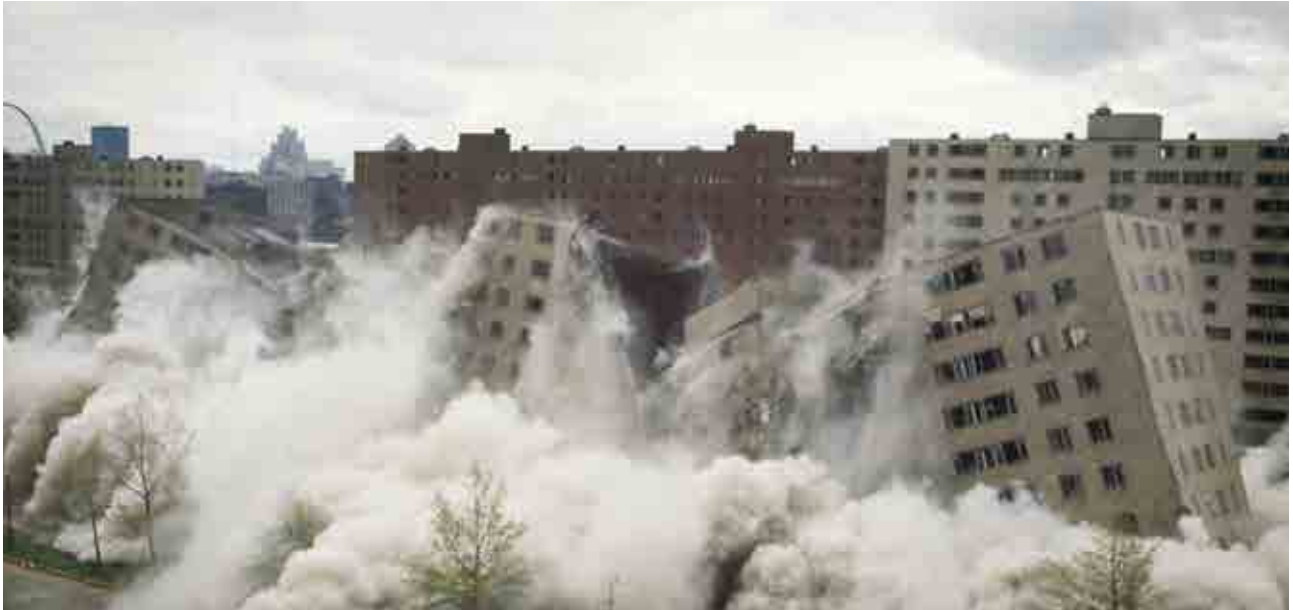
The Pruitt-Igoe housing project in St Louis, US, built according to Modernist planning concepts, was demolished just 18 years after construction
