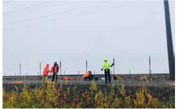
Figure 3: Geophysical survey (ERA) by Norwegian PhD students (Karlis Riekst&Vadim Simonsen) with Russian railway engineering staff (Alexander Kekelev) supervised by MSU geophysist (Oleg Komarov).
