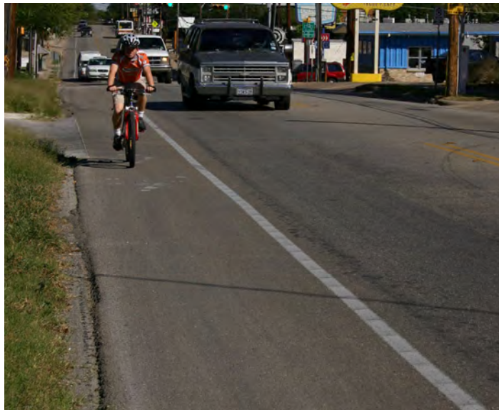
Figure 7.5. Example of an uneven seam between the gutter pan and roadway (grass is covering the curb face)
