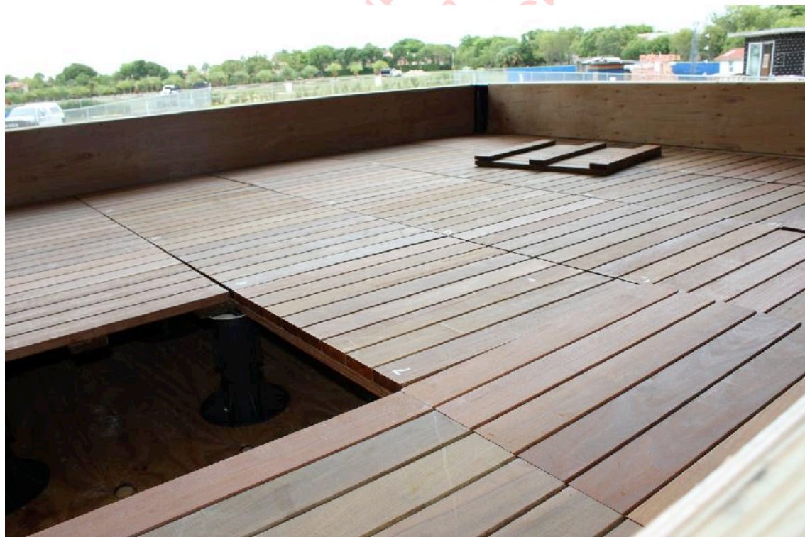
Figure 7 - Paver blown off into the leeward parapet
