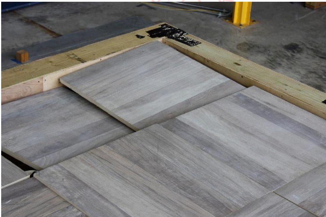
Figure 15 - Pavers pushed down into the windward corner of the roof by the wind.
