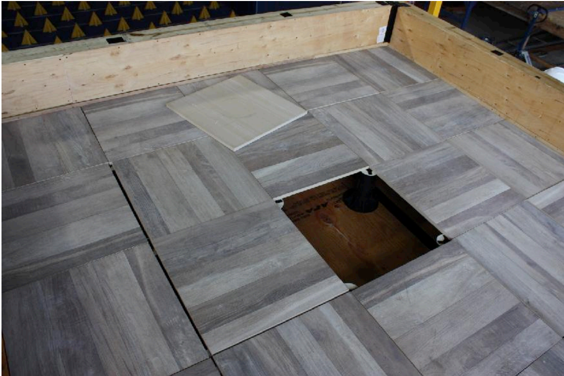
Figure 12 - Porcelain paver flipped upwards by the wind.
