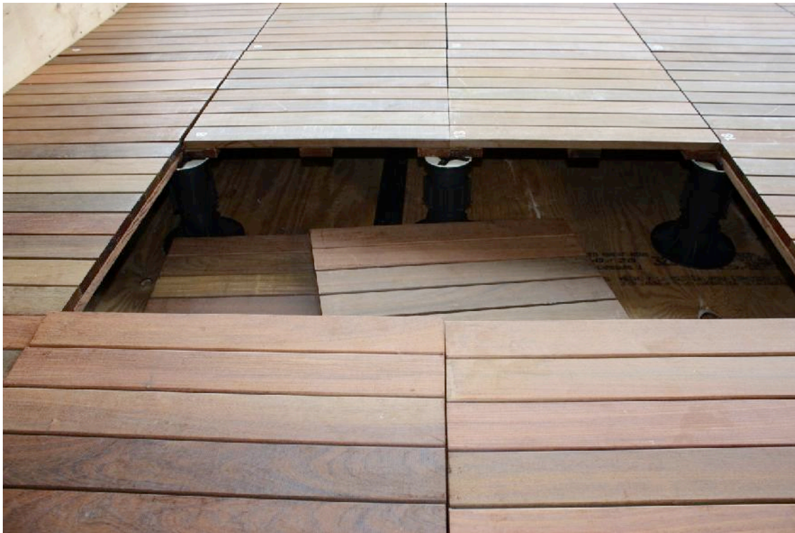
Figure 6 - Pavers blown off pedestals; wind picked them up but didn't blow them off the roof. As they set down they fell onto the roof deck pushing away some of the adjacent pedestals
