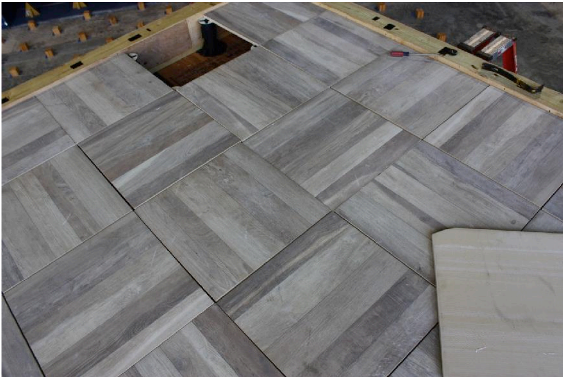
Figure 14 - Porcelain paver blown off by the wind from its location along the perimeter of the windward edge of the roof. A chipped corner may be seen on the paver from when it hit down.
