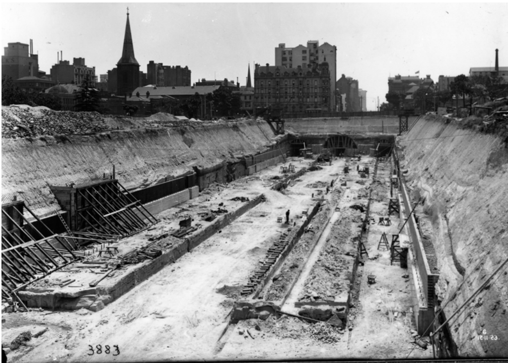
St James Station under construction looking towards Macquarie Street. St James Church, after which the station was named, is to the left. Note that there was no need to excavate the section where the platforms would be as it would only have to be filled up again!
