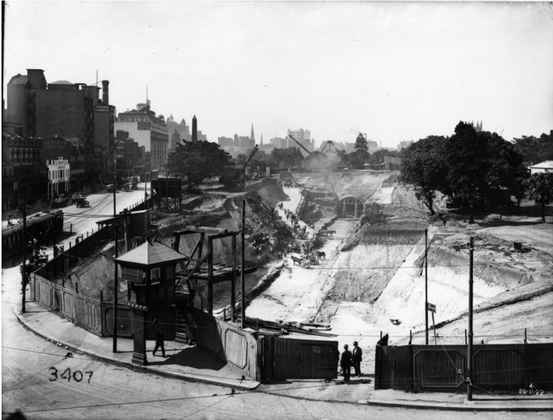
Museum Station under construction looking from the corner of Elizabeth Street and Liverpool Street towards the centre of Hyde Park. The tramway signal box is not at the Sydney Tramway Museum at Loftus.
