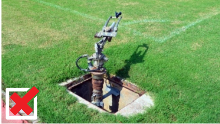
Metal cover too near corner mark
