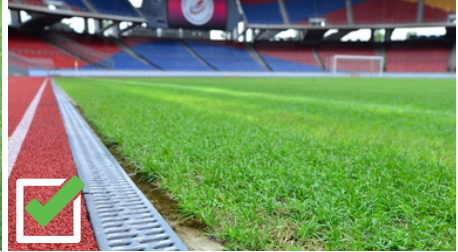
Proper drainage cover
