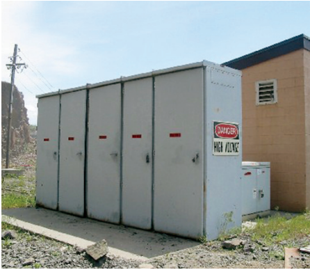
5 kV medium voltage lineup
