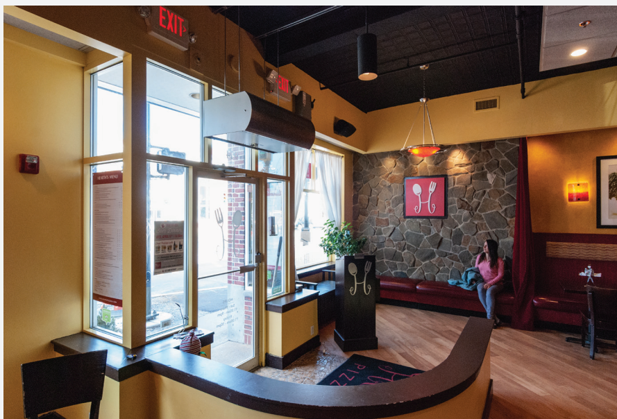
Berner Architectural High Performance 10 Air Curtain on Customer Entrance
