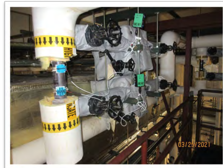
EverActive Sensors installed at 3M Brookings
