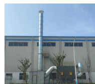
Fume Treatment Equipment
