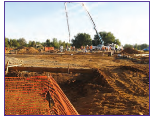
The first of the concrete flowed into the "E" wing, where rooms for our Veterans will soon take shape.
