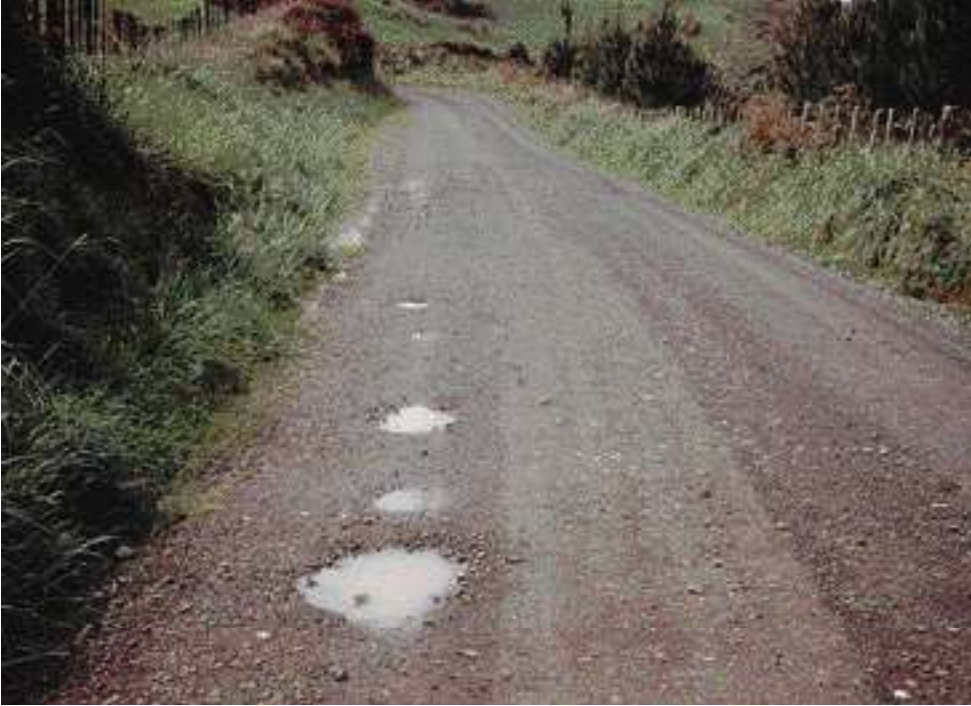
This road located in New Zealand does not have adequate crown to drain water to the roadside. Consequently, potholes form. (Courtesy of Ken Skorseth, SD LTAP)
