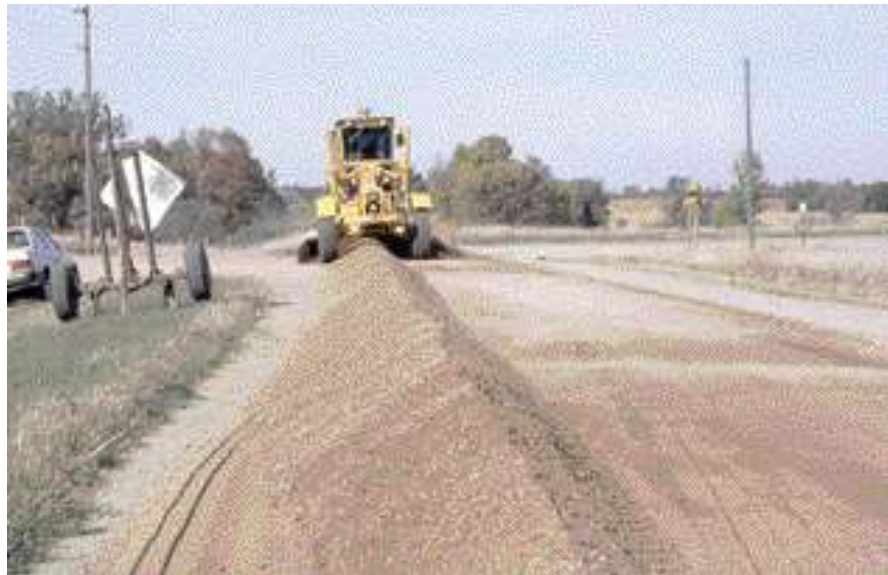
Only after completely windrowing and equalizing does the operator begin to place the material at a uniform depth across the roadway.
