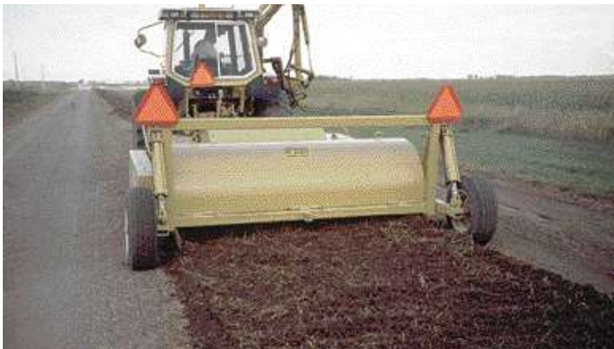
A machine fabricated specially by Hyde County in South Dakota to pulverize heavy windrows of recovered gravel and grass from the shoulder. It quickly breaks down windrows for reuse on the road.
