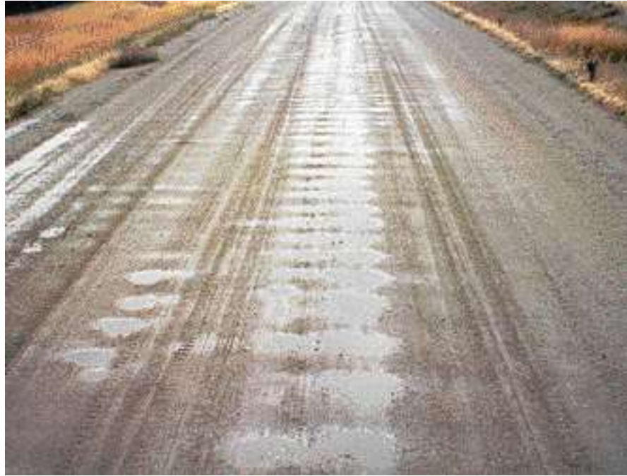
A road that lacks good crown. There is also centerline corrugation (washboarding), a problem that will grow worse when there is inadequate crown.
