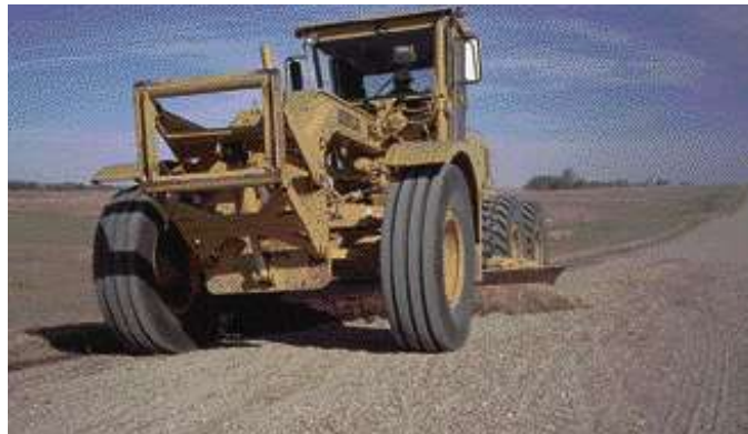
The existing surface gravel is cut loose and windrowed to the opposite side of the road.
