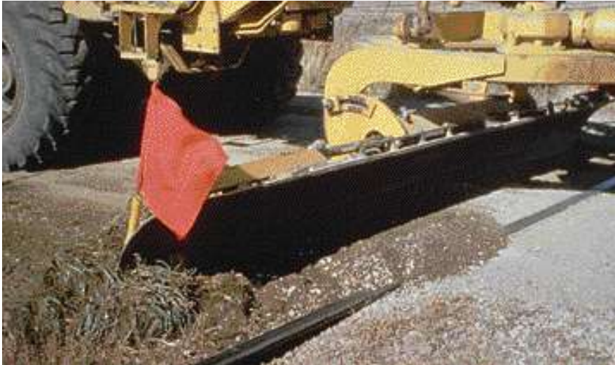
Grader working at a rural railroad crossing. The material that has been pushed into the flange-way should be removed.
