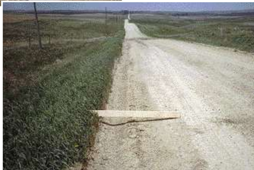
Secondary ditch over six inches deep.
