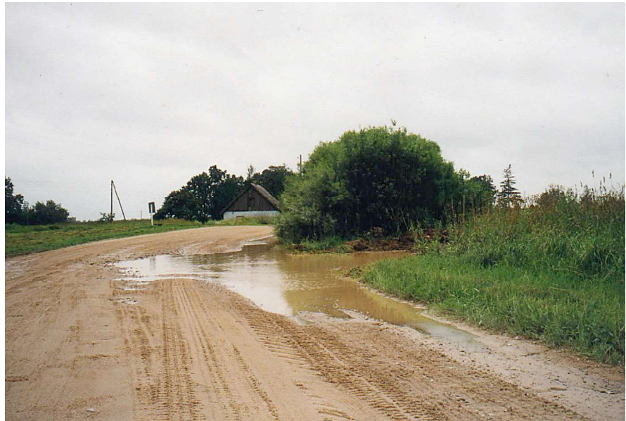
Lack of a roadside ditch has caused major drainage problems on this road.(Courtesy of Road Research Ministry of Roads/Transportation,Sweden)
