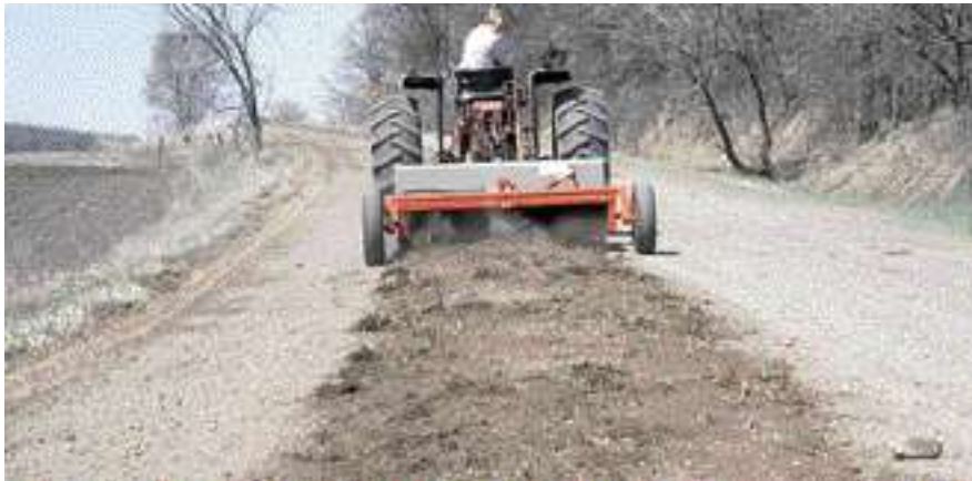
A machine made in Canada pulverizes gravel windrows into usable material on the roadway.
