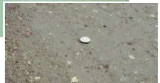
Notice the good blend of stone, sand and fine-sized particles tightly bound together on this road surface.
