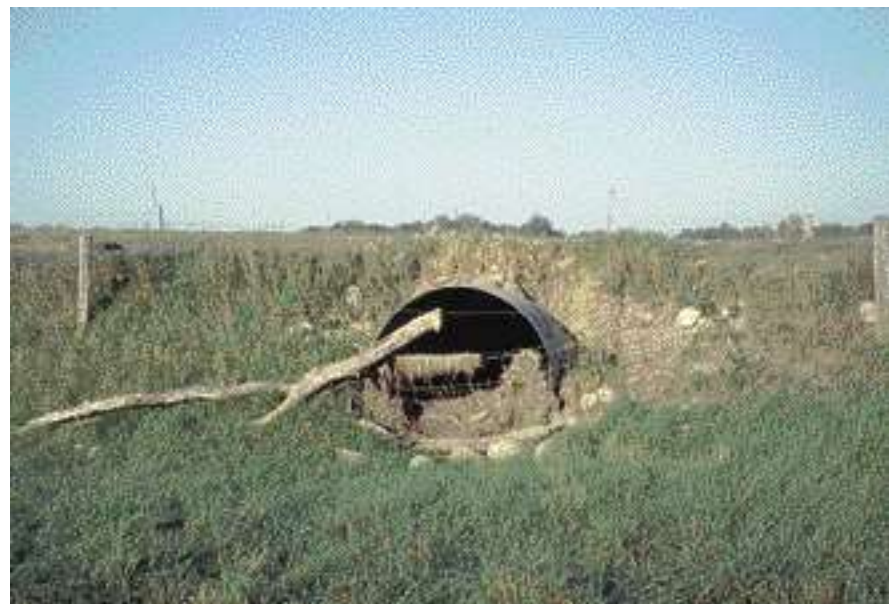
This road could fail if debris is not cleared before the next heavy rain.
