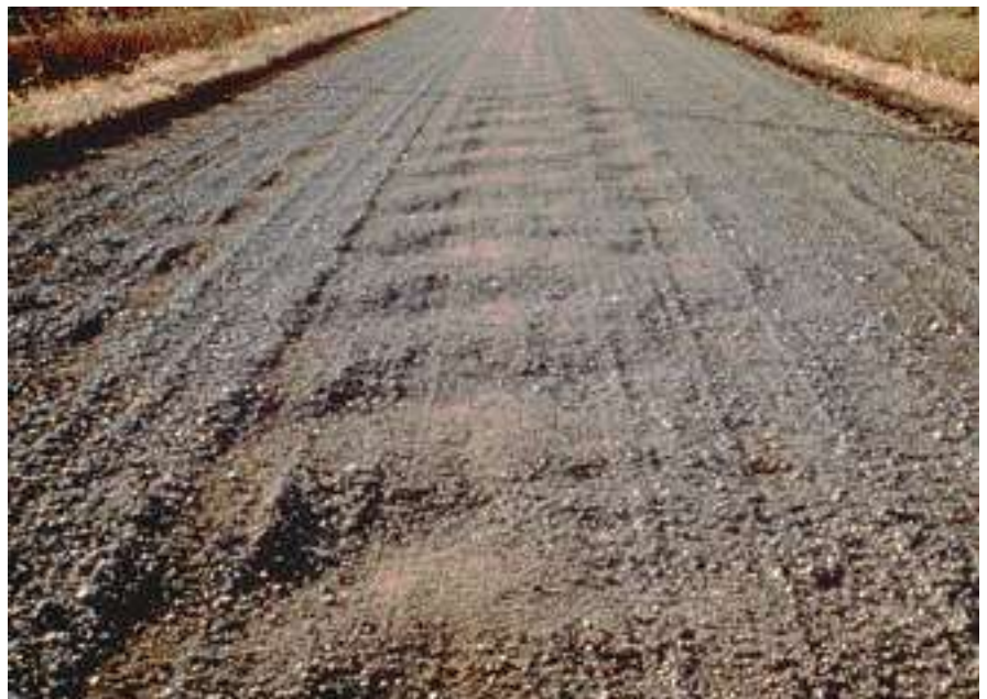
This type of washboarding appears at an angle across the roadway with ridges and depressions two to three feet apart. It is caused by excess grader speed.
