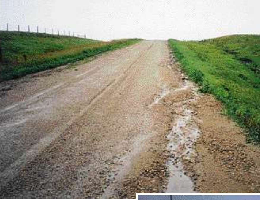
A common condition along the edge of many gravel roads: the secondary ditch.
