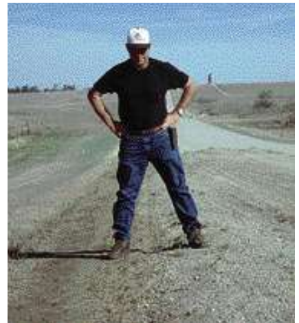
The windrowed gravel is then brought back over the recovered material and the roadway is restored to proper crown and shape. The high shoulder has been eliminated.
