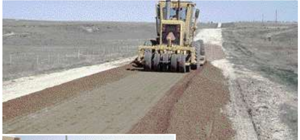
A grader-mounted roller being used on a rural gravel road. This department owns three of these units.
