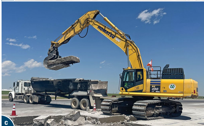
Steve Waalkes, Michigan Concrete Association, used with permission (a); Resonant Machines, LLC, used with permission (b); ACPA, used with permission (c)
